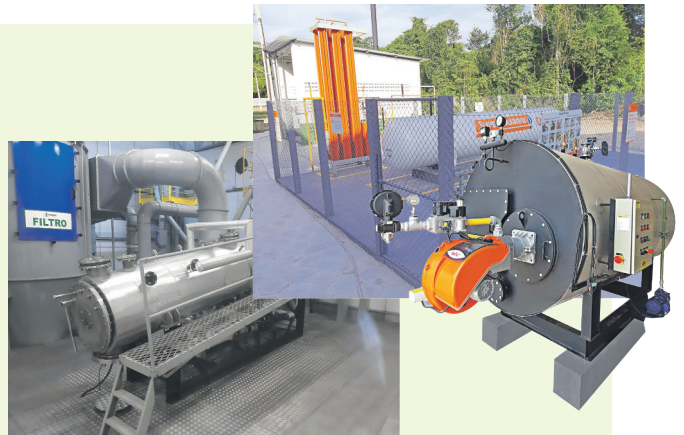
Purchase and installation of machinery for steam sterilization of black pepper, including gas supply station, boiler, and dryers.
